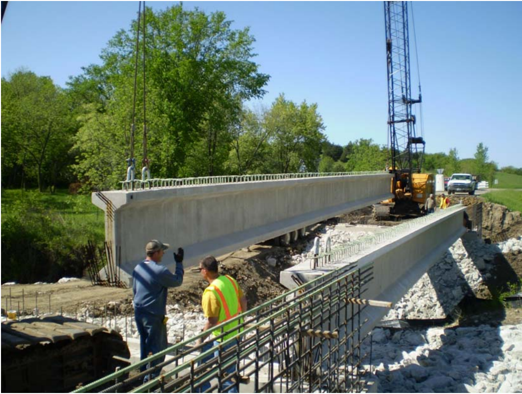
Prestressed concrete girders are being set on Route AA for a bridge replacement in Clark County
